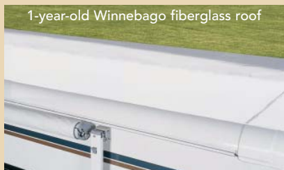
1-year-old Winnebago fiberglass roof
