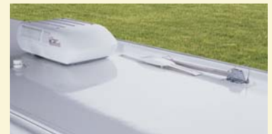
One-year-old Winnebago Industries fiberglass roof
