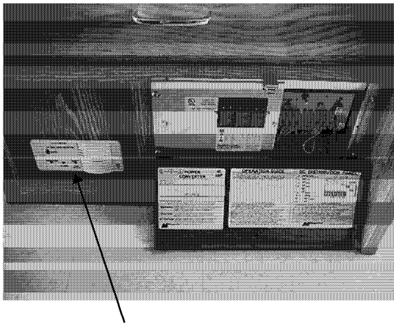
LP Gas Alarm
