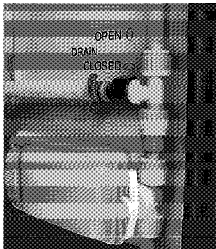
Water Line Drain in right front compartment
