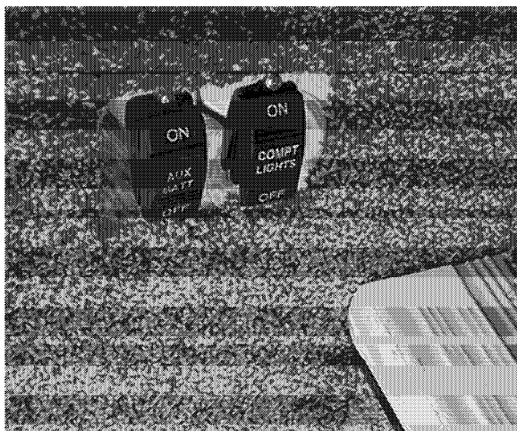
Aux. Batt. Switch (Near entrance door)
