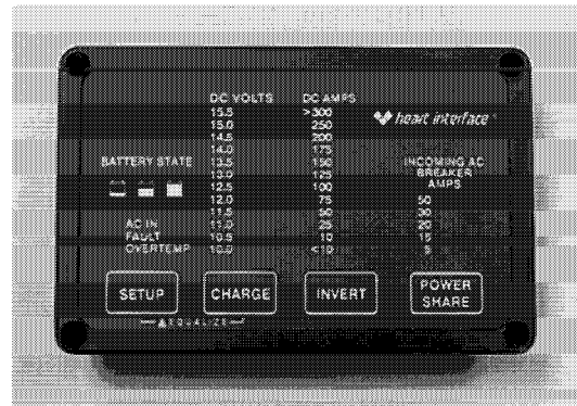
Inverter Charger Control Panel
