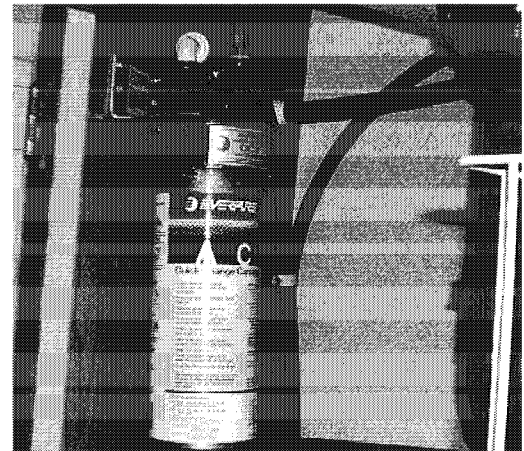
Water Filter Assembly - Below Galley Sink
