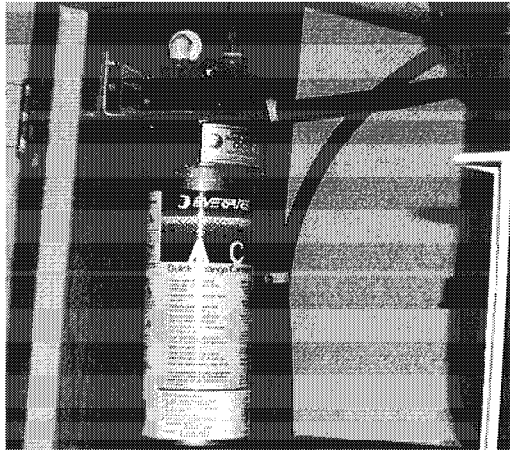
Water Filter Assembly - Below Galley Sink
