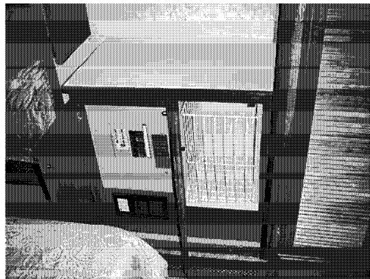
House 110-Volt Breaker Panel in Bedroom Closet
