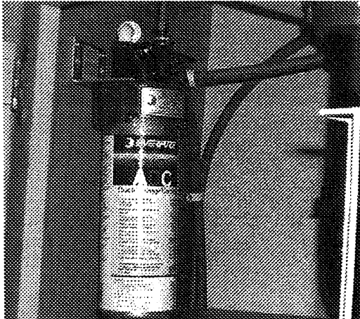
Water Filter Assembly - Below Galley Sink
