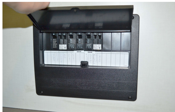
120-Volt Circuit Breakers -Typical View
