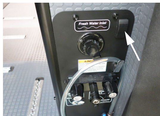
Pump switch -Typical View
