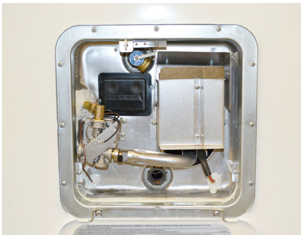
Water Heater Exterior Service Access
