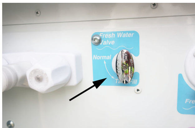
Fresh Water Valve in tank fill position (Located in water service center) -Typical View
