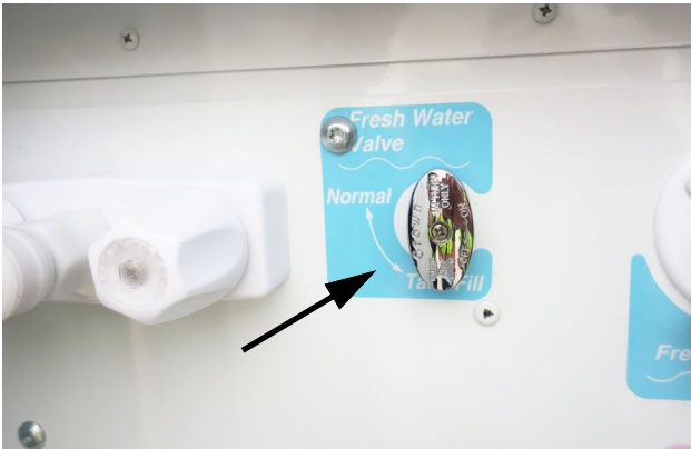
Fresh Water Valve in tank fill position (Located in water service center) -Typical View
