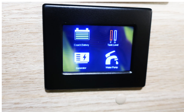
System Monitor Panel -Typical View
