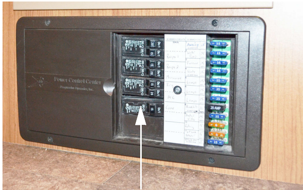
120-Volt Circuit Breakers -Typical View
