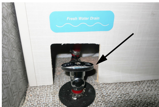
Close the 1 General Waterline drain- Passenger Side Compartment Drain Valve (Shown in the closed position). -Typical View
