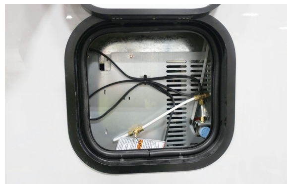
Refrigerator Access Door (open) -Typical View
