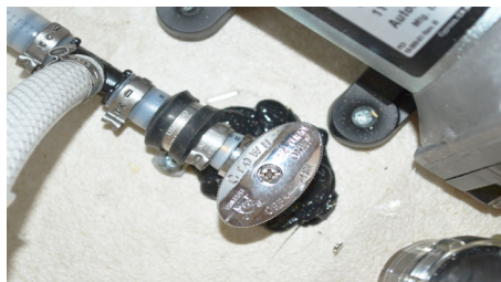
Water Tank Drain Valve -Typical View
