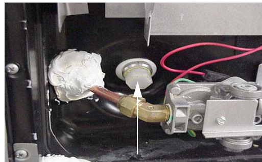
Water Heater Drain Plug (Remove with socket)
