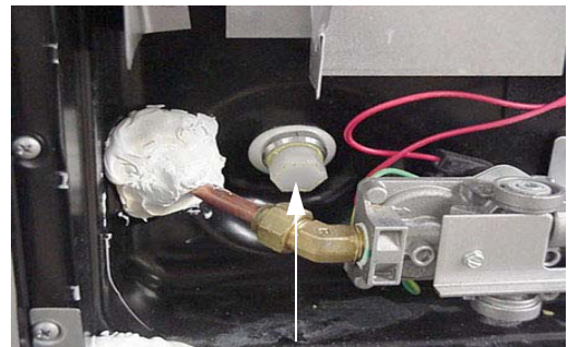
Water Heater Drain Plug (Remove with socket)
