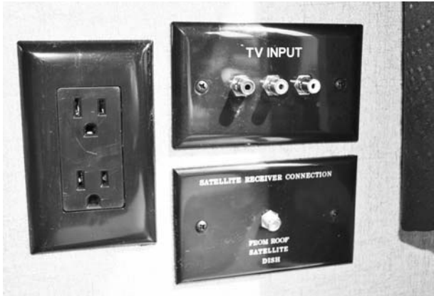
Bedroom DVD/Satellite Receiver Connection -Typical View
