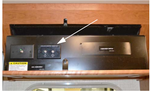
Interior Connection for Satellite Dish -Typical View
