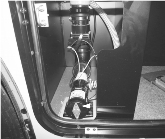
Waste Pump (Located in passenger side compartment ahead of rear axle) -Typical installation shown
