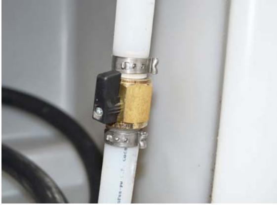
Water Tank Drain Valve -Typical installation shown
