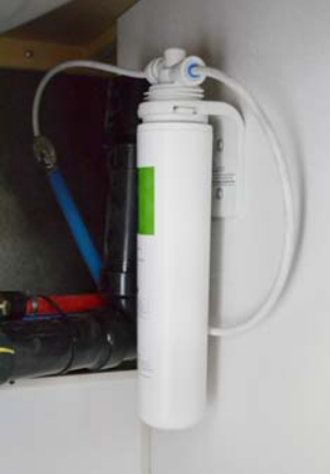
Ice Maker Water Filter Assembly (Located below galley sink)
