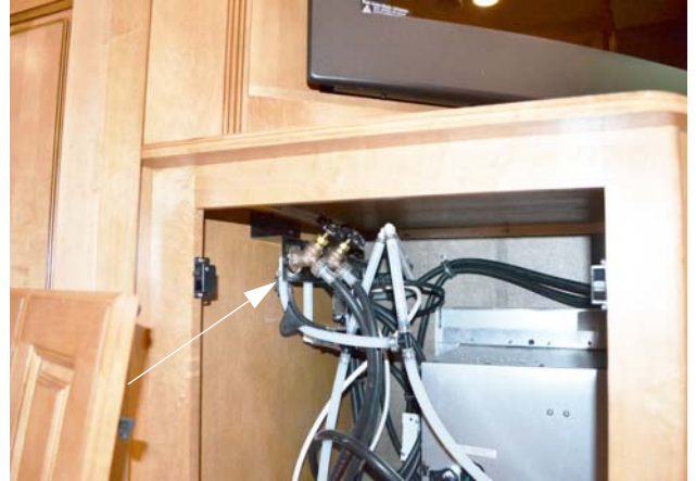
Water Supply Faucets (Located behind access panel in bedroom TV/Fireplace cabinet)
