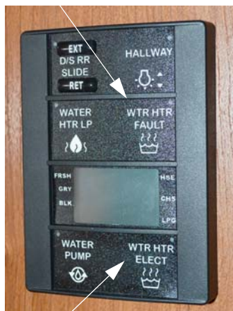
Electric Water Heater Switch (Located on Systems Monitor Panel) -Typical View
