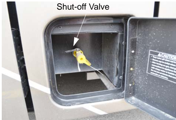
LP Accessory Connection (Located behind lockable access door on passenger side of coach) -Typical View
