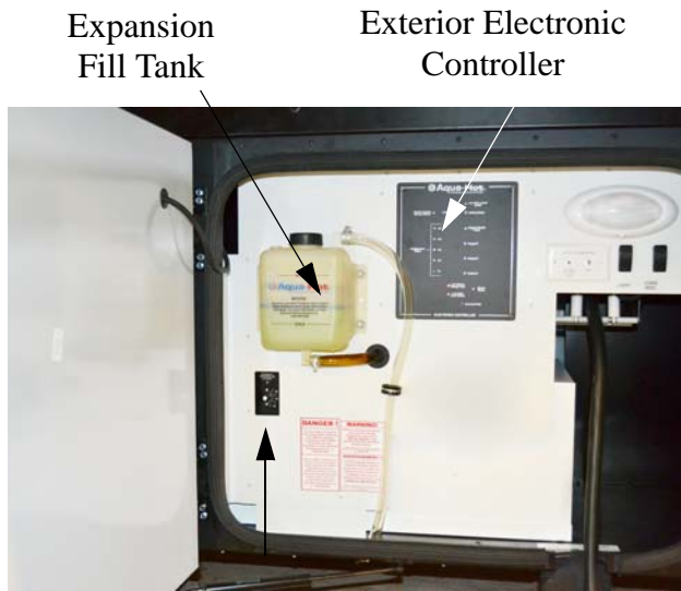
Basement Temperature Control
