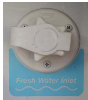
Fresh (City) Water Connection “Fresh Water Inlet” (Located in the water service center) -Typical View
