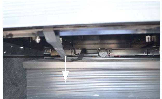
Emergency Retract Strap (Located underneath stepwell cover) Typical View
