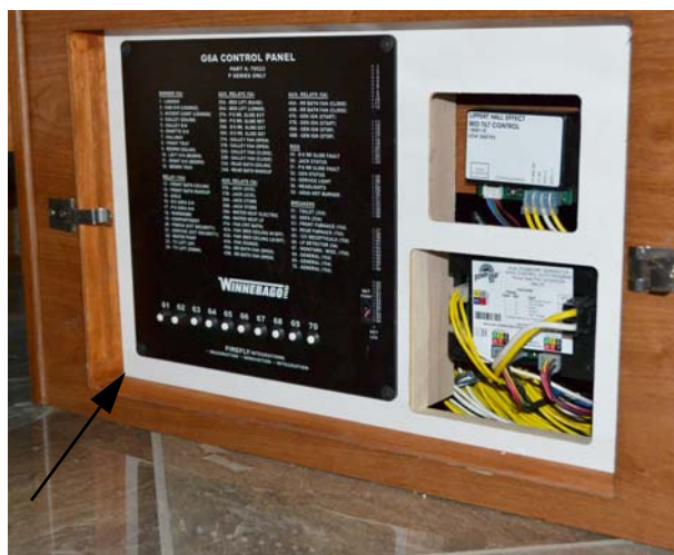
House Circuit Breakers -Typical View
