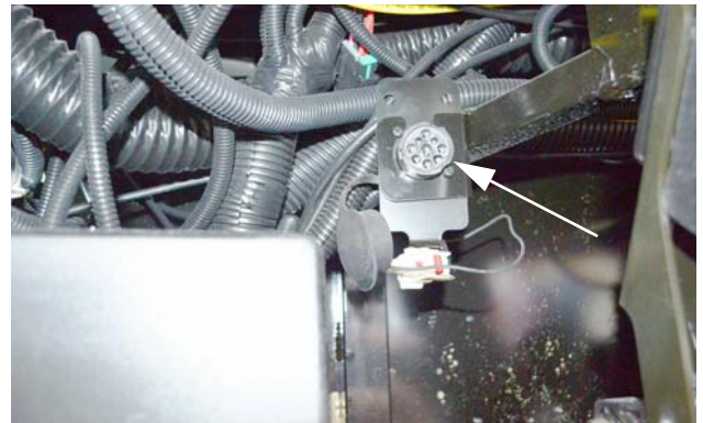
Diagnostic Plug (Located on steering column support beneath left side of dash) -Typical View
