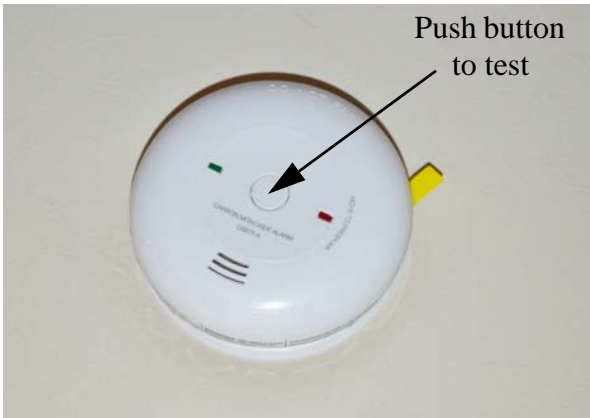
Carbon Monoxide Alarm
