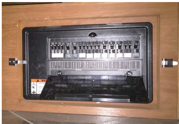
House Circuit Breakers -Typical Installation
