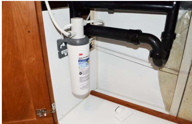
Galley Filtered Cold Water Faucet/ Ice Maker Filter Assembly (Located below galley sink) -Typical View
