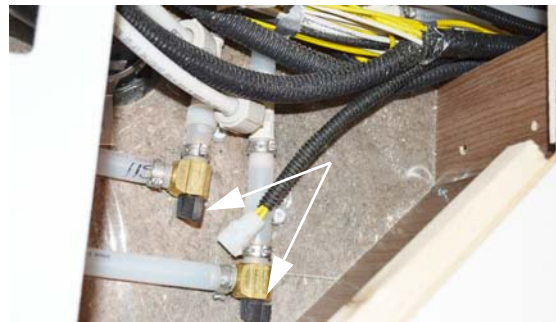
Waterline Drain Valve
