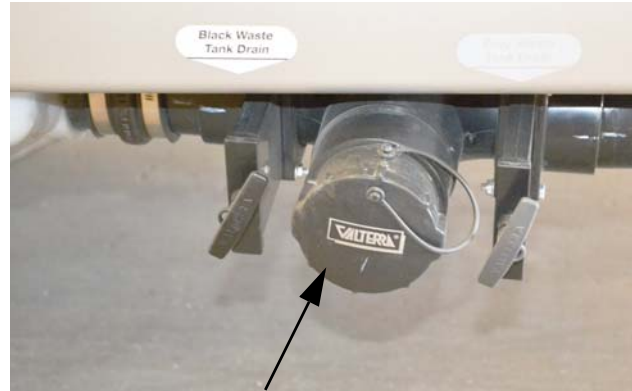
Sewage Drain Outlet (Located on the underside of water service center) -Typical View
