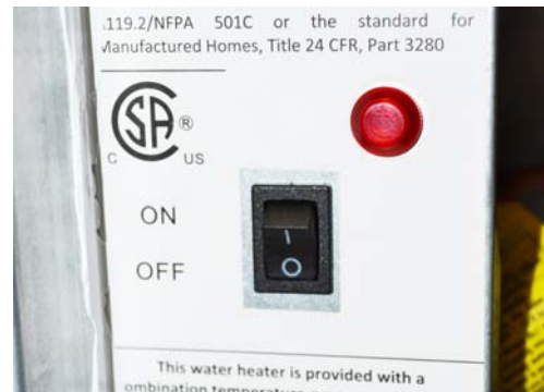
Water Heater (Tankless) Power Switch
