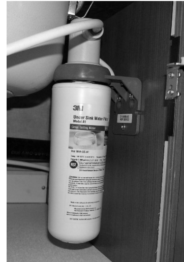
Cold Water Filter Assembly (Located below galley sink) NOTE: Hot waterline is not filtered.
