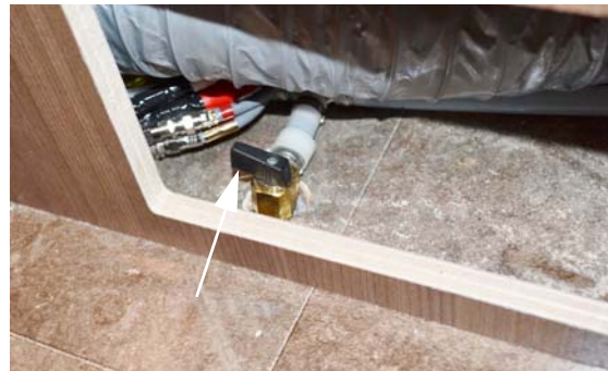
Water Tank Drain Valve
