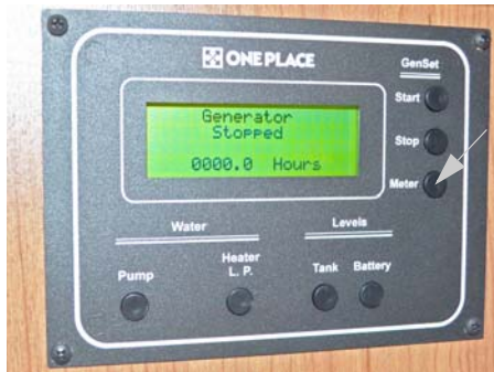
Generator Hourmeter Button -Typical View
