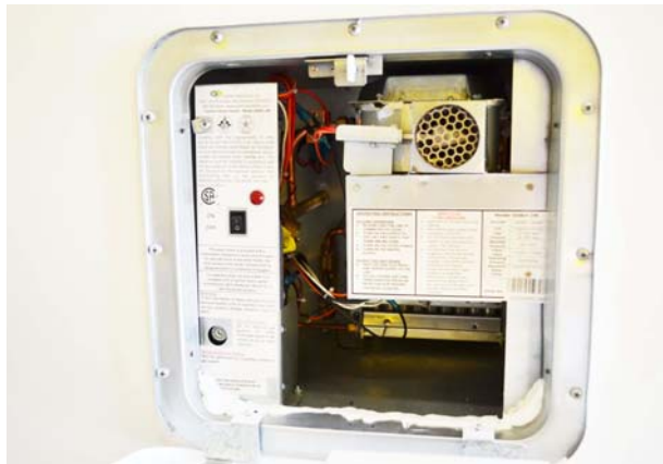
Water Heater Exterior Service Access -Typical View
