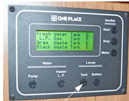
Tank Levels Switch
