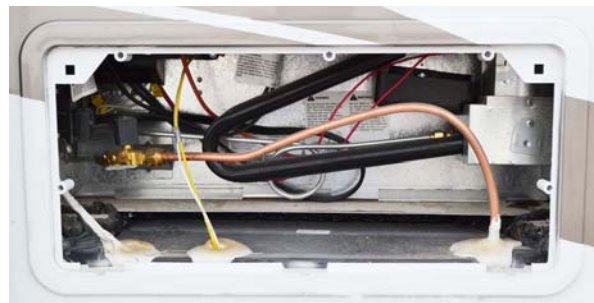
Refrigerator Access Compartment -Typical View
