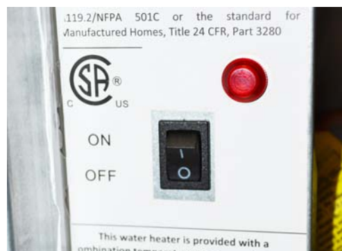
Water Heater (Tankless) Power Switch
