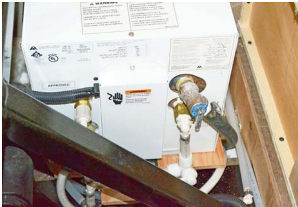
Water Heater Interior Service Access (located below forward facing dinette seat) -Typical View
