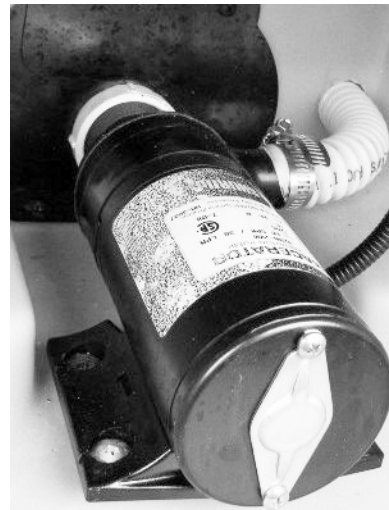
Waste Pump (Located beneath coach) -Typical View
