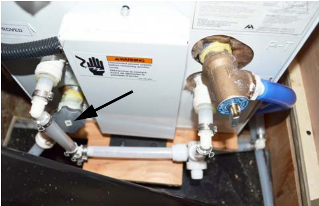
Water Heater Drain Plug
