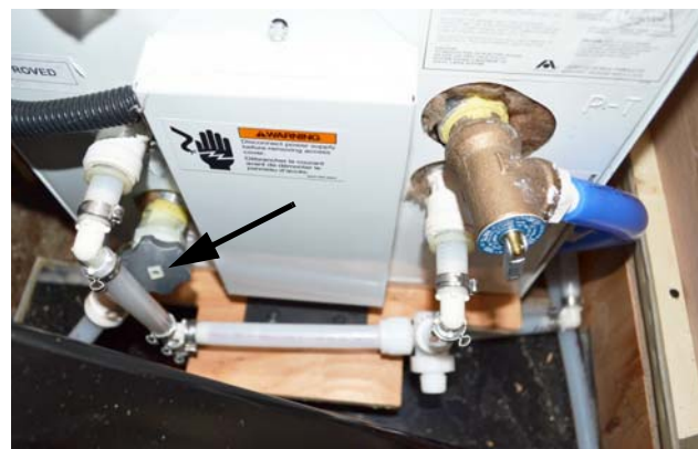
Water Heater Drain Plug
