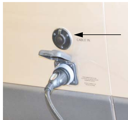
Cable TV Input Connection (Located on the left sidewall)
