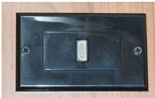
HDMI Connection (Located in cabinet behind TV) -Typical View
