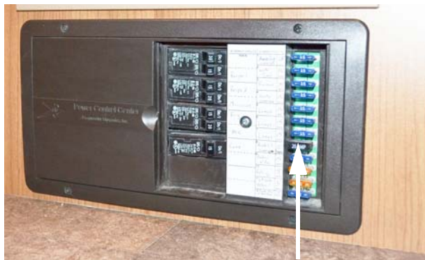
House 12-Volt Fuses (Located on right-hand side of Power Converter) -Typical View
