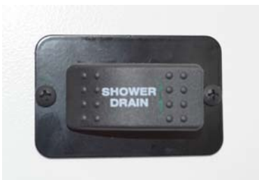
Shower Drain Switch (Located near shower head) -Typical View
