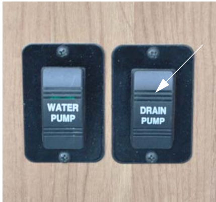
Waste Pump Switch (Located in the water service center)
