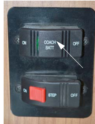
House/Coach Battery Disconnect Switch (Located on galley end) -Typical View
