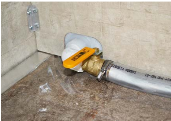
Water Tank Drain Valve OFF -Typical installation shown
