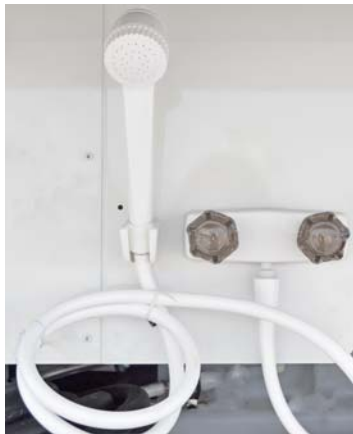
Exterior Shower/Wash Station -Typical View
