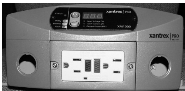
Inverter Unit (Located inside an exterior compartment) -Typical View
