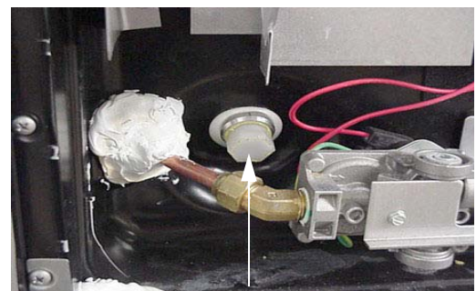
Water Heater Drain Plug (Remove with socket)
