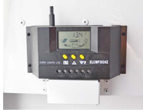
Solar Charge Controller (Located in utility compartment)
