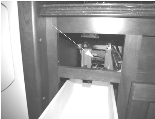
Water Supply Faucets (Located beneath rear bath lavatory cabinet)
