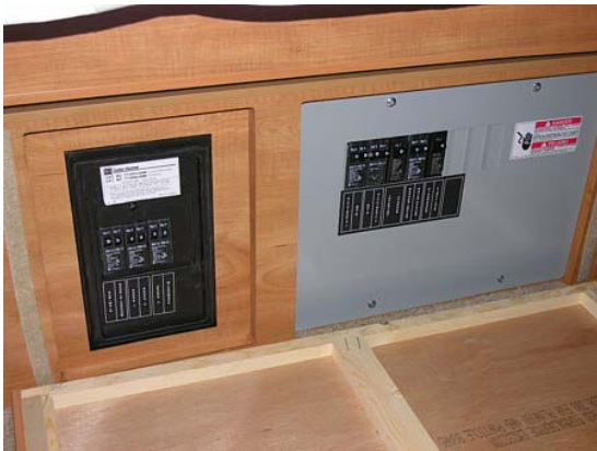
House Circuit Breakers -Typical Installation
