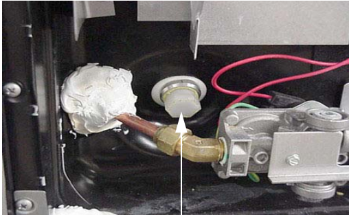
Water Heater Drain Plug (Remove with socket)
