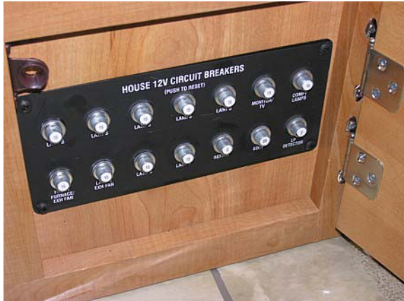
House Circuit Breakers -Typical View
