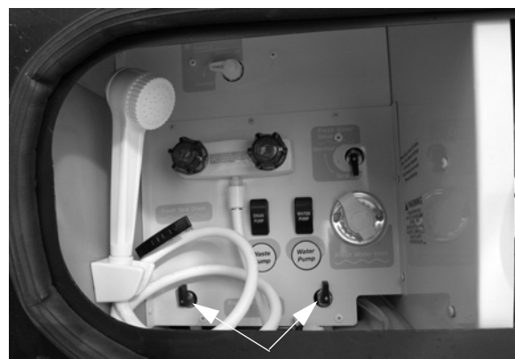
Waterline Drain Valves -Typical View
