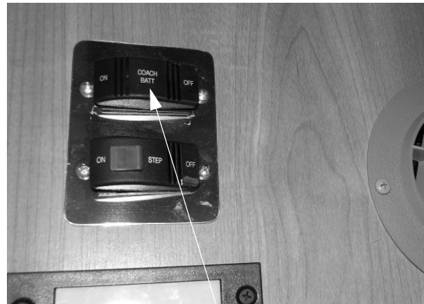
House/Coach Battery Disconnect Switch (Located near entrance door or end of galley, depending on model) -Typical View
