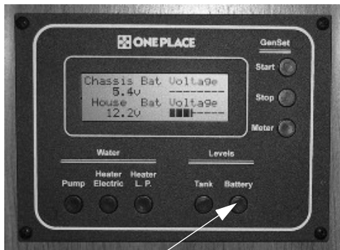
Battery Levels Switch
