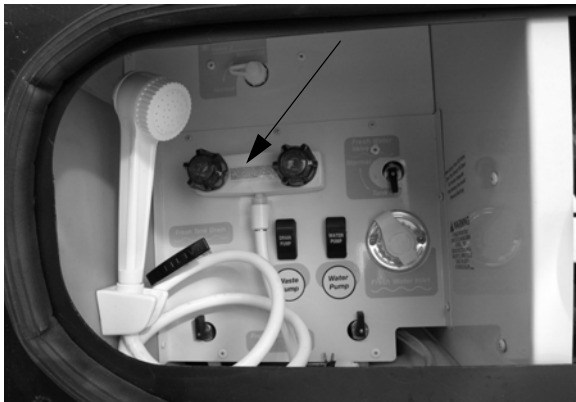
Exterior Shower/Wash Station (Located in water service center) -Typical View
