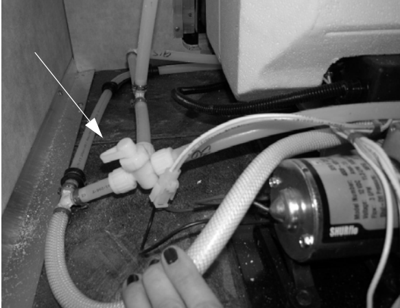
Water Heater Bypass Valve
