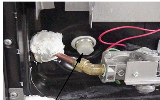
Water Heater Drain Plug (Remove with socket)
