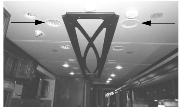
Supply/Return Air Vents (Located throughout the ceiling of the coach) * View looking to rear of coach
