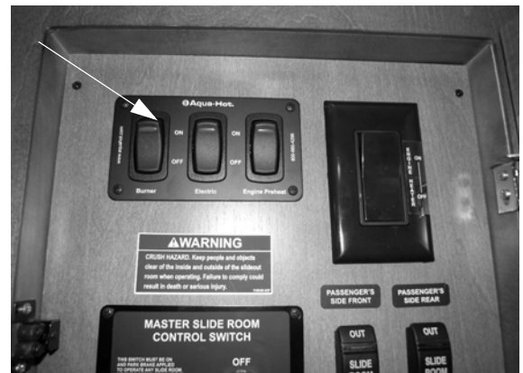
Hydronic Heating System Interior Control Switches (Located near monitor panel) -Typical View
