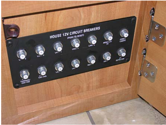
House Circuit Breakers -Typical View
