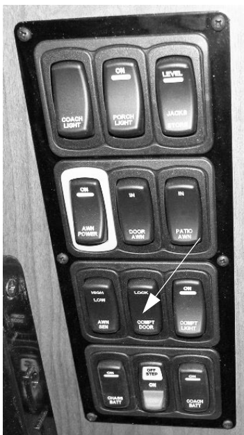
Power Door Locks - Compartment Doors (Located on entry switch panel) -Typical View
