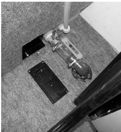
Water Tank Drain Valve (Located in first passenger side compartment) -Typical View
