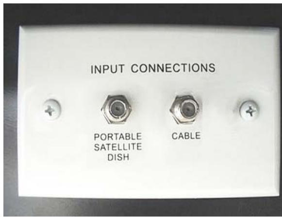
Exterior Connection for Satellite Dish and Cable TV (Located in the shoreline compartment)
