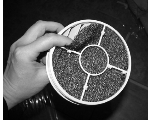
Air Filter (Located on back side of Return Air Vent) -Typical View
