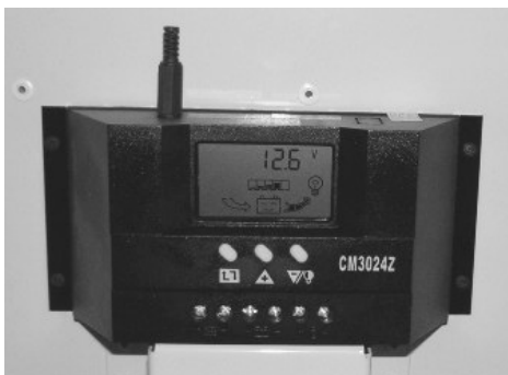
Solar Charge Controller (Located in utility compartment)
