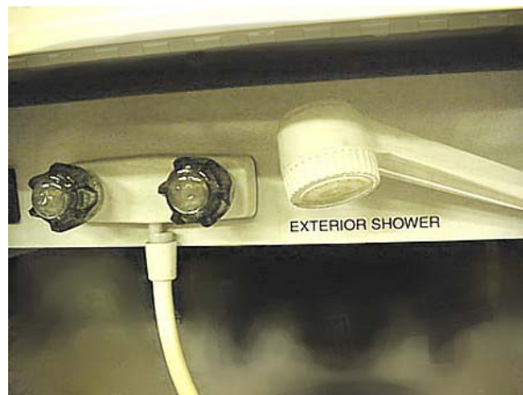
Exterior Shower/Wash Station -Typical View
