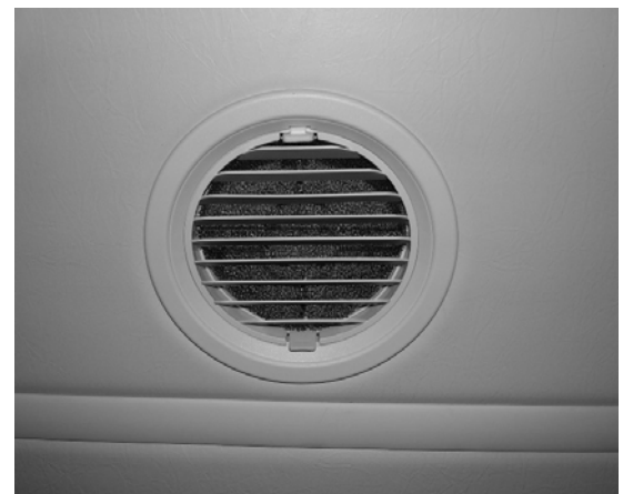
Return Air Vent (Shown with filter installed) -Typical View
