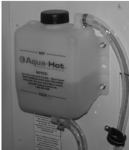
Expansion Fill Tank
