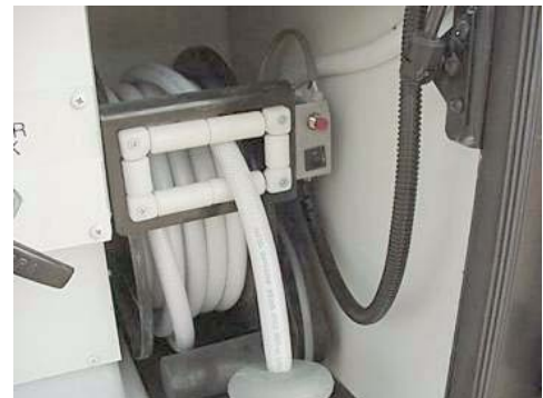
Water Hose Reel (Located in the water service center) -Typical installation shown
