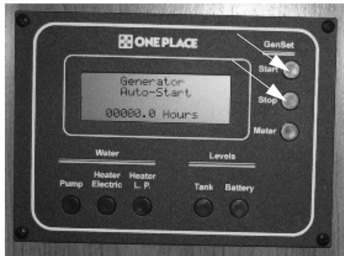
LP Generator Start/Stop Buttons (Located on monitor panel) -Typical View
