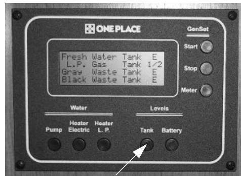
Tank Levels Switch
