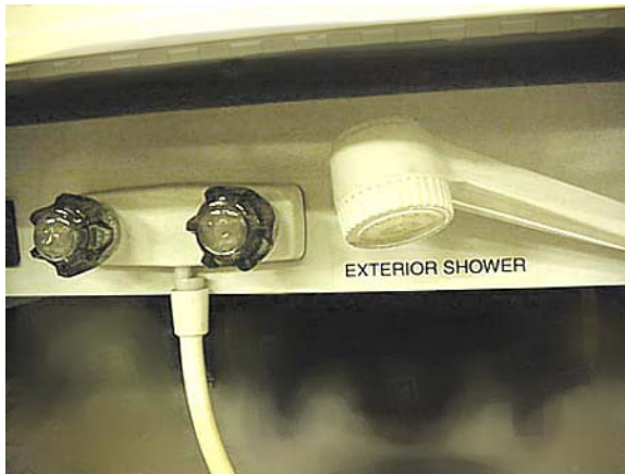
Exterior Shower/Wash Station -Typical View
