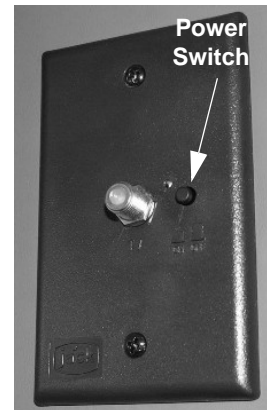
TV Signal Amplifier Power Switch (Located near entertainment center cabinet) -Typical View
