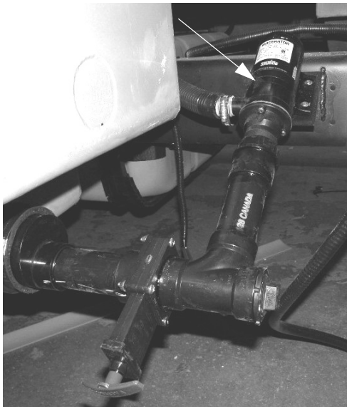
Waste Pump (Located on driver side of coach behind rear wheel) -Typical View
