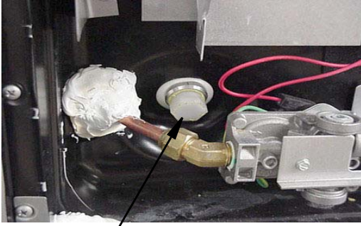
Water Heater Drain Plug (Remove with socket)
