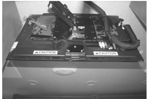
Entrance Door TV (View shown from entrance step)
