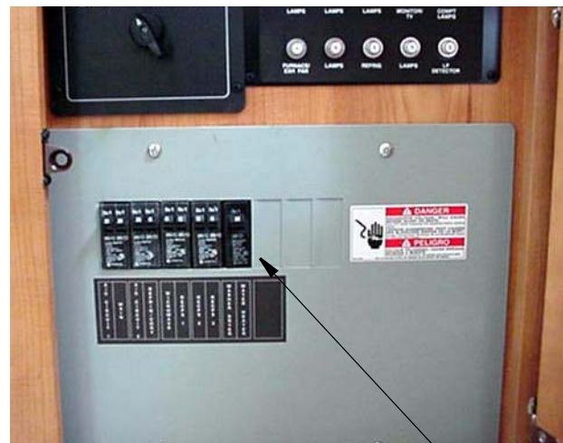
120-Volt House Circuit Breakers -Typical View
