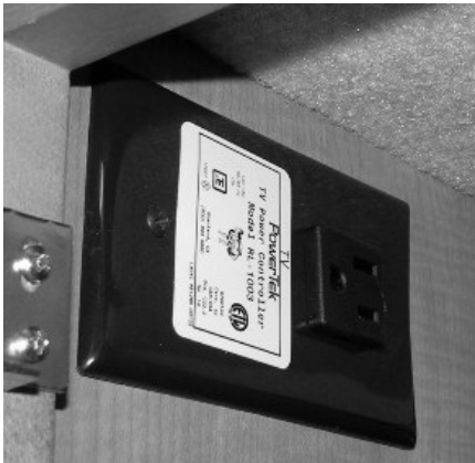
Front TV Ignition Switch Interlock -Typical View
