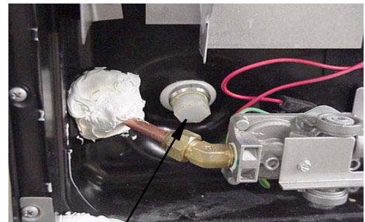
Water Heater Drain Plug (Remove with socket)
