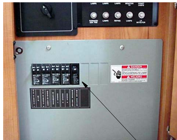
120-Volt House Circuit Breakers
