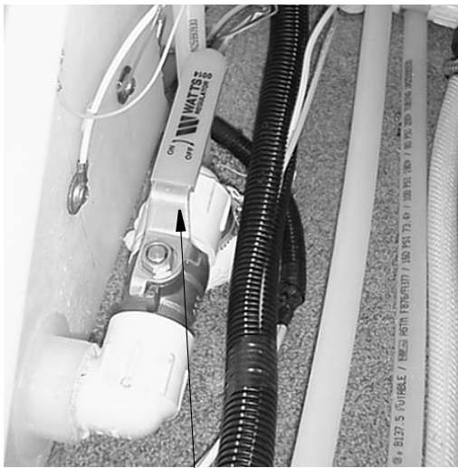
Water Tank Drain Valve (Typical)
