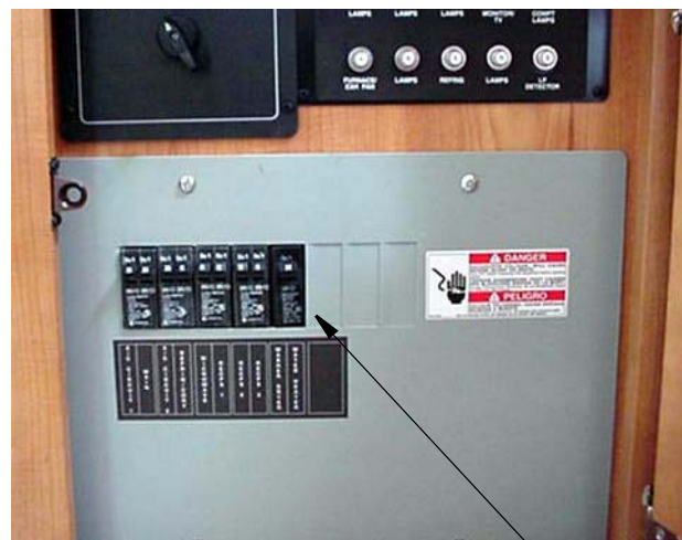
120-Volt House Circuit Breakers
