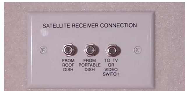
Interior Connection for Satellite Dishes (in overhead cabinet near TV*)
