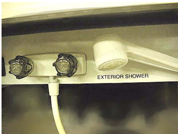
Exterior Shower/Wash Station (typical)
