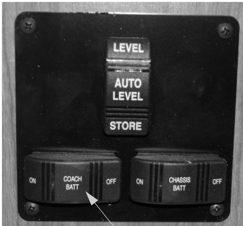
Auxiliary Battery Switch - Typical (Near Entrance Door)
