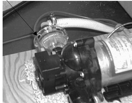
Water Pump and Filter
