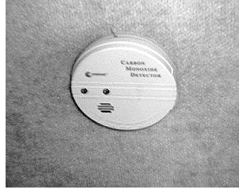
Carbon Monoxide Alarm
