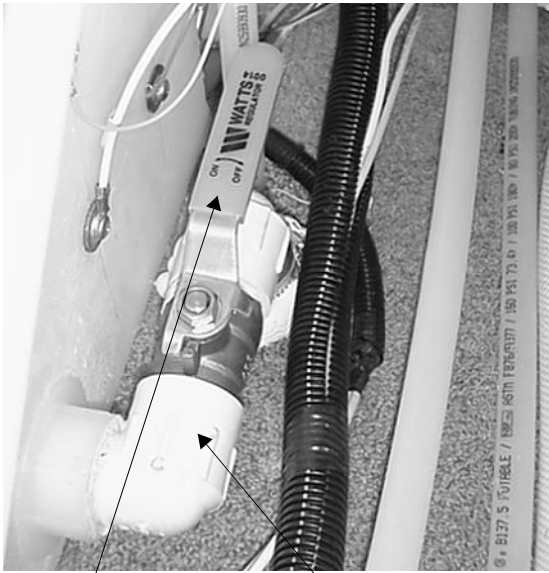
Water Tank Drain Valve Winterization Valve
