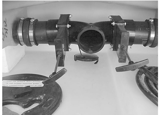
Holding Tank Dump Valves
