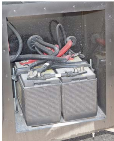
Chassis Batteries (Located in a rear driver side compartment) -Typical View
