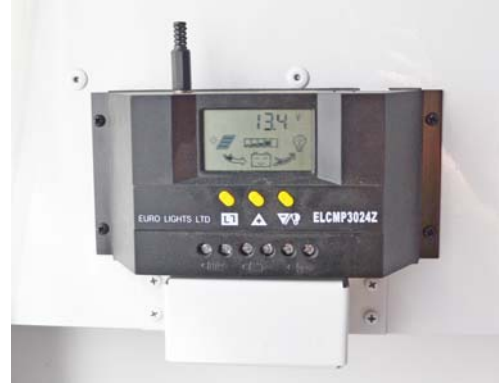
Solar Charge Controller (Located in utility compartment)
