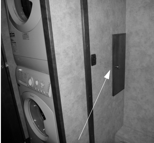
Water Supply Faucets (Located behind access door within the rear wardrobe)
