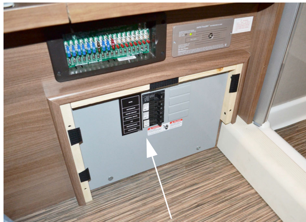
120-Volt Circuit Breakers -Typical View
