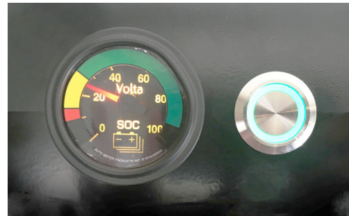
Pure 3 State of Charge (SOC) Gauge (Located on an interior cabinet) -Typical View
