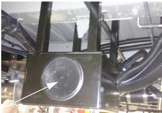
Waste Pump Enclosure (Located beneath motorhome)
