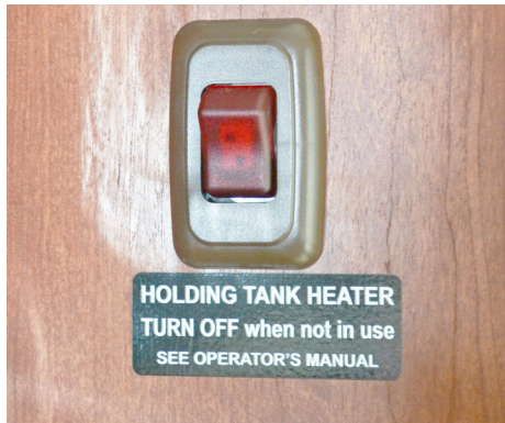
Tank Heater Switch (Located near monitor panel) -Typical View
