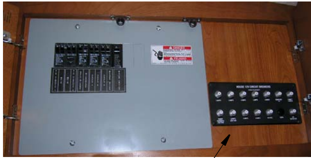
House 12-Volt Circuit Breaker Panel
