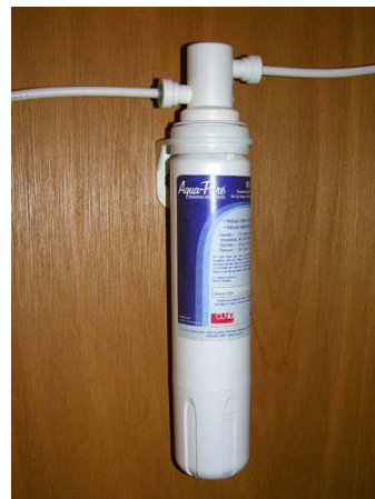
Water Filter Assembly below Galley Sink
