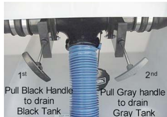
Holding Tank Dump Valves (Typical)
