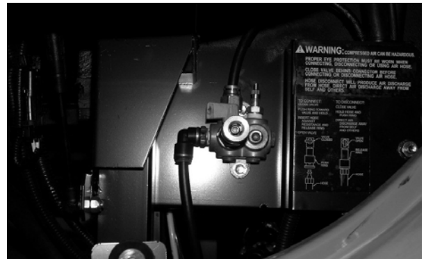
Quick Connect Air Coupler and Air Valve at front end of coach
