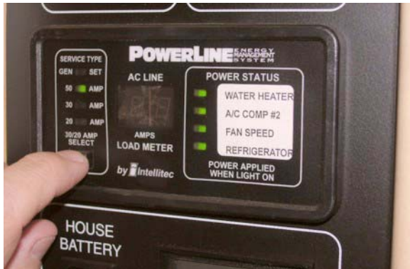
PowerLine EMS Display on Monitor Panel - Typical
