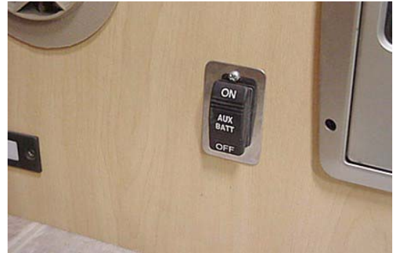
Aux. Batt. Switch - typical (Near entrance door)
