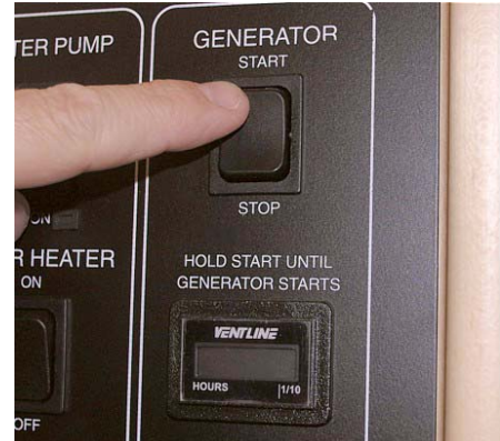
Generator Switch and Hourmeter on monitor panel
