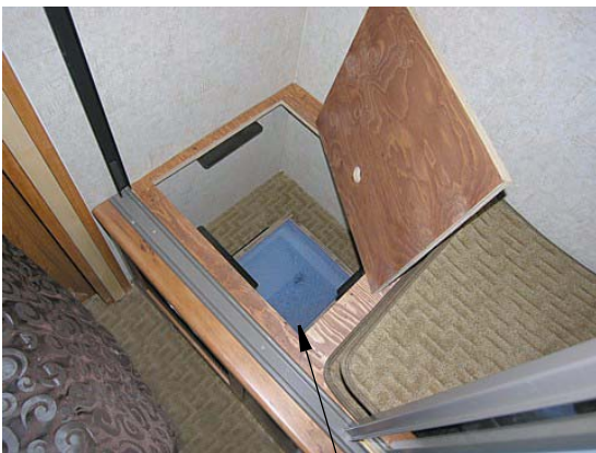
AC/Furnace Filter under wardrobe floor panel
