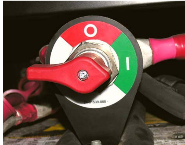
Diesel Chassis Battery Cutoff Switch inside battery storage compartment
