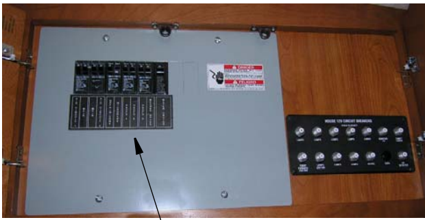
House 120-Volt AC Circuit Breaker Panel
