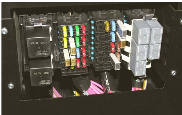
Automotive Fuses (Cover Removed) - Diesel
