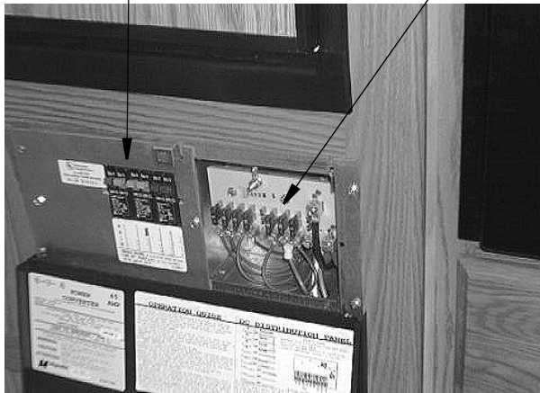
Power Center (Converter)
