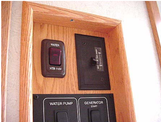
Diesel Engine Heater Switch
