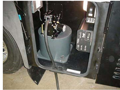
Inverter Charger Unit Location in shoreline compartment
