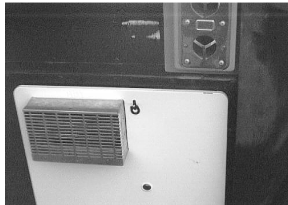
Water Heater Service Access Panel
