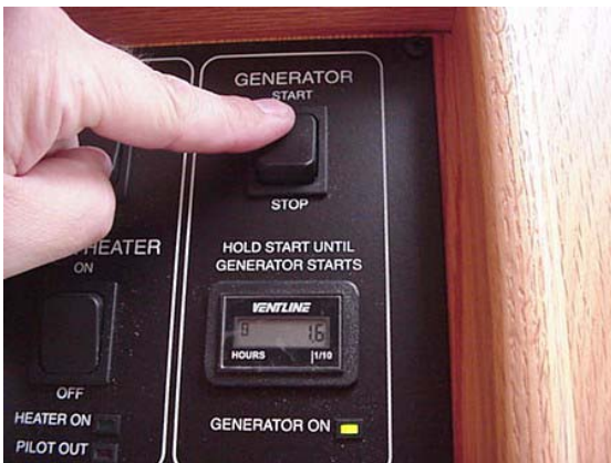
Generator Switch and Hourmeter
