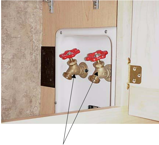
Water Supply Faucets Typical
