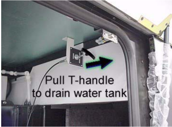
Water Tank Drain Valve (pull to open)
