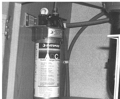
Water Filter Assembly - Below Galley Sink
