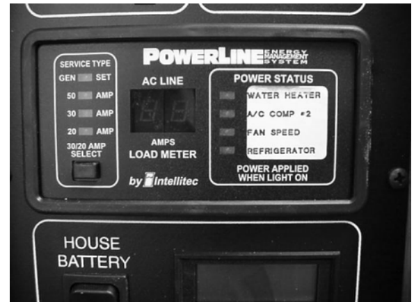
EMS Display on OnePlace Monitor Panel
