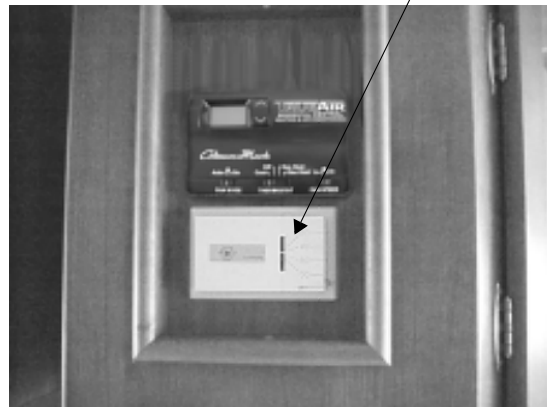
Power Ventilator Thermostat - Galley
