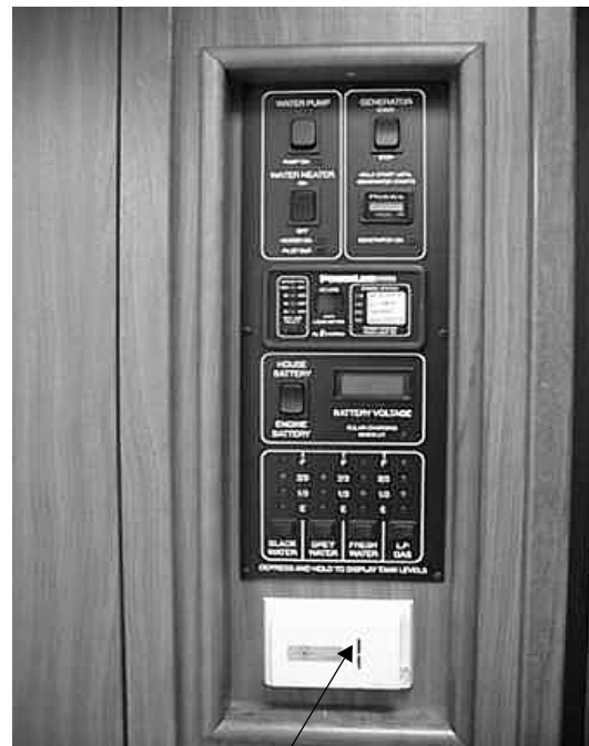
Power Vent Thermostat Bath Area
