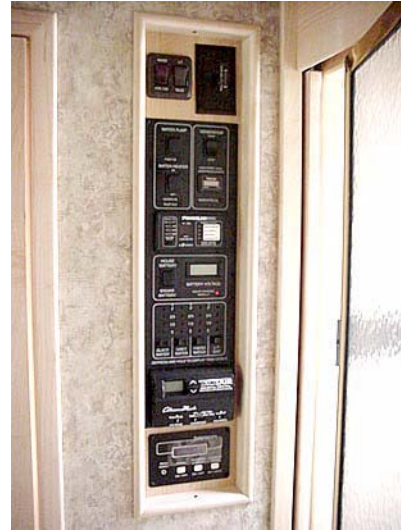
One Place Monitor Panel
