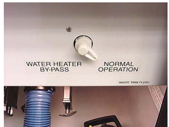
Water Heater By-Pass Valve (Typical)
