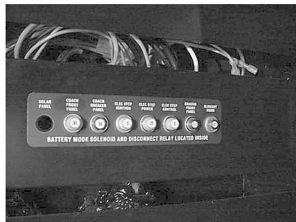
Chassis and House 12V Circuit Breakers in cargo compartment near entrance door
