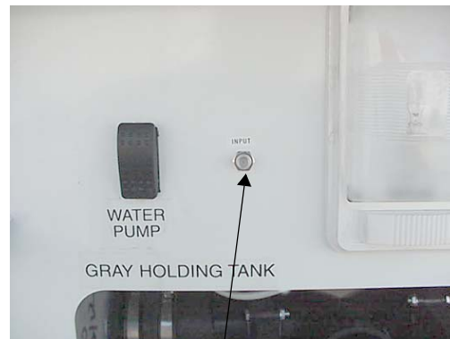
Cable TV Hook-Up in Utility Compartment
