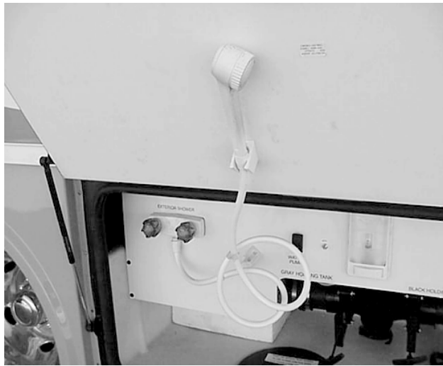
Exterior Shower/Wash Station (Typical)
