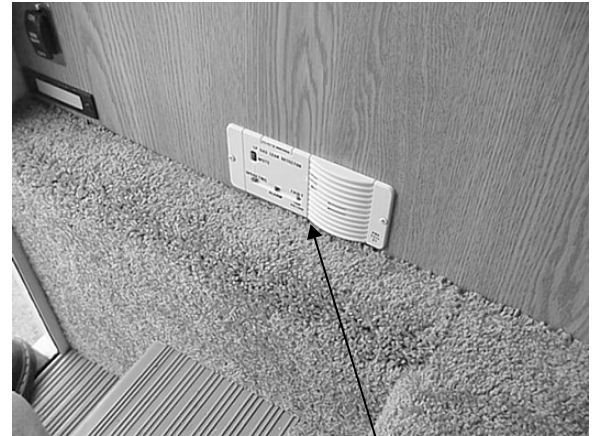
LP Gas Alarm
