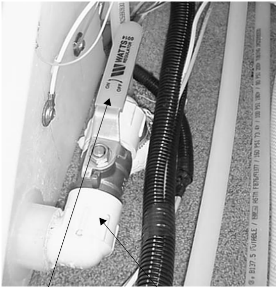
Water Tank Drain Valve Winterization Valve
