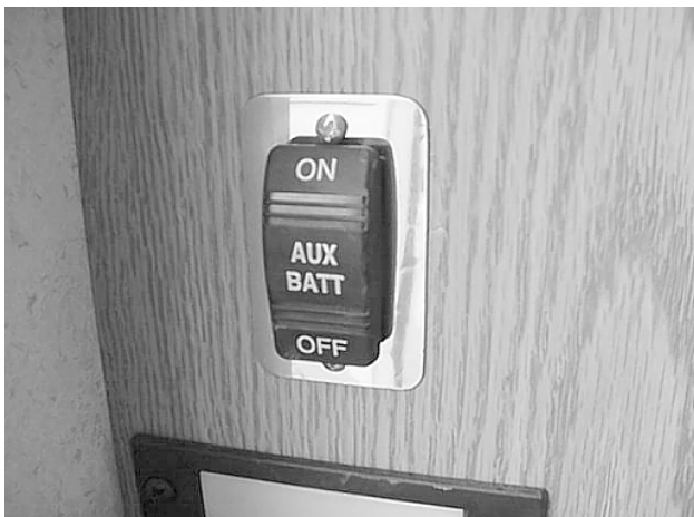
Aux. Batt. Switch (Near entrance door)
