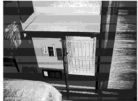
House 110-Volt Breaker Panel in Bedroom Closet
