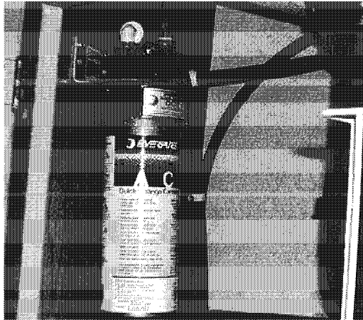
Water Filter Assembly - Below Galley Sink
