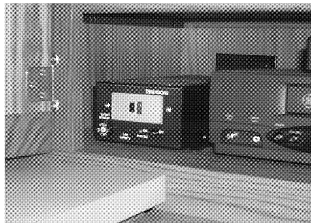
DC-AC Voltage Inverter in Video Center
