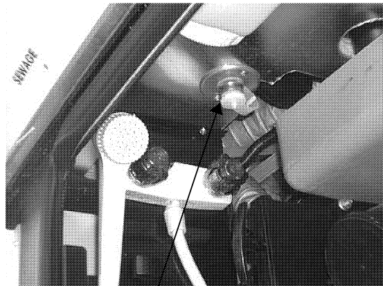
City Water Connection
