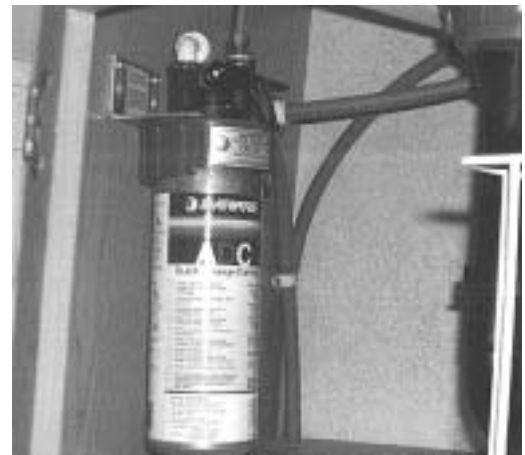
Water Filter Assembly - Below Galley Sink
