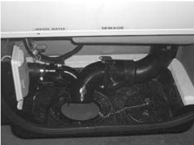
Holding Tank Dump Valves
