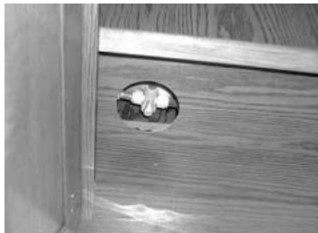
Water Heater By-Pass Valve (Typical) Beneath Galley Sink
