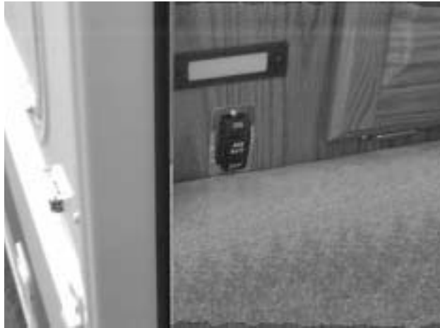
Aux. Batt. Switch (Near entrance door)
