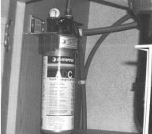
Water Filter Assembly - Below Galley Sink
