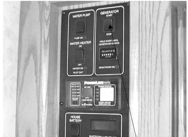
Generator Switch and Hourmeter
