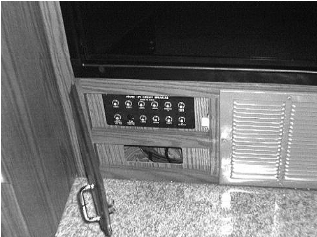
House 12V Breakers (below refrigerator)
