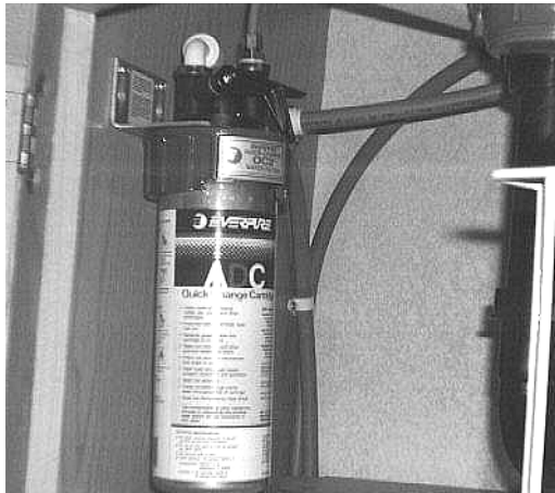
Water Filter Assembly - Below Galley Sink
