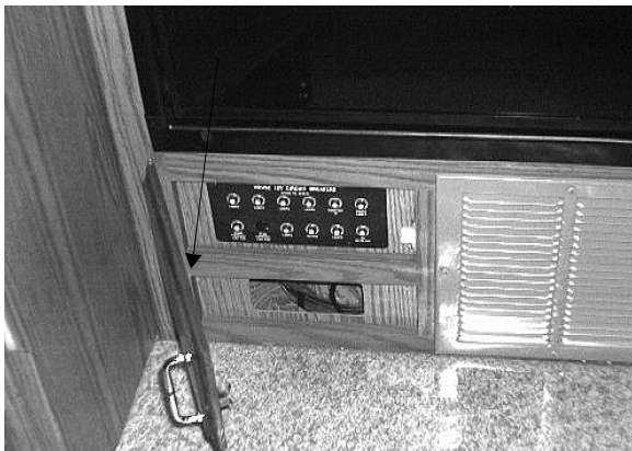
House 12-Volt Circuit Breaker Panel
