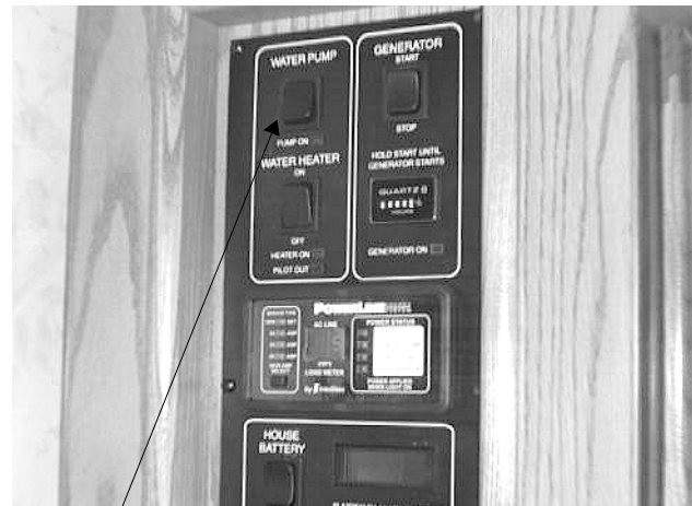
Water Pump Switch
