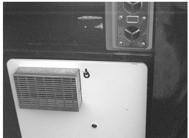
Water Heater Service Access Panel
