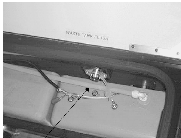
Flushing System Inlet
