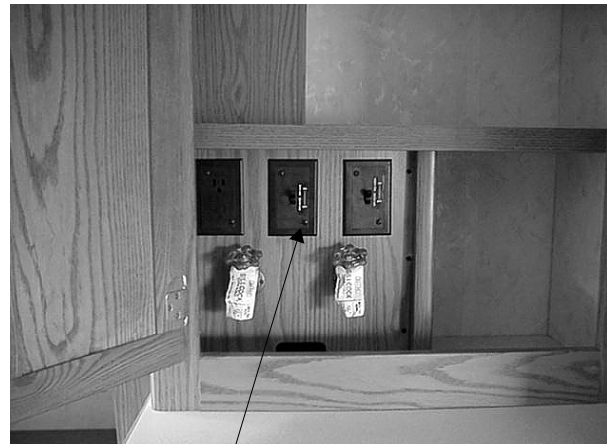
Water Heater Switch Electric Operation
