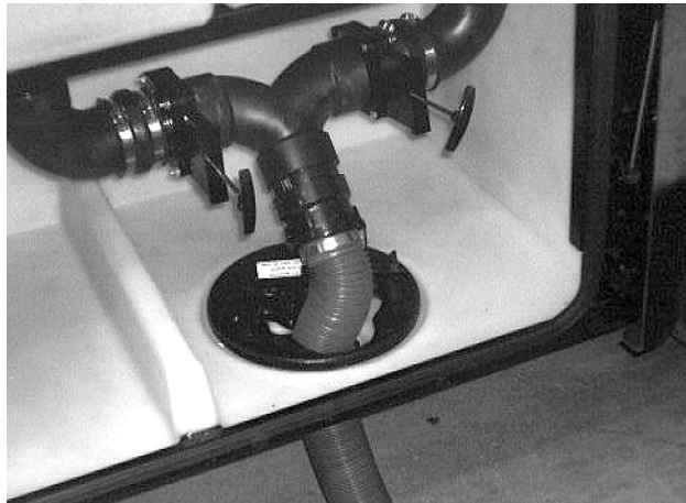
Drainage Hose routed through passage in compartment
