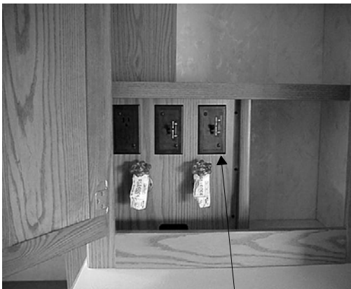
Engine Block Heater Switch In Cabinet to Right of Medicine Chest
