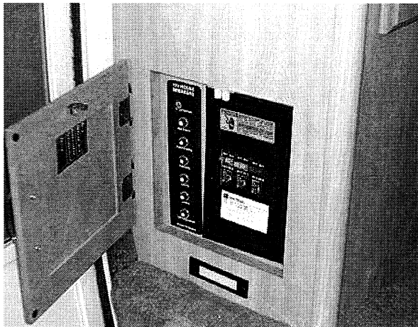
12-Volt Breaker Panel - Model 22FD
