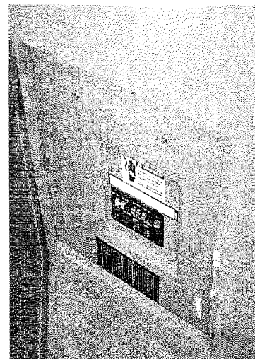
House 110-volt Breaker Panel
