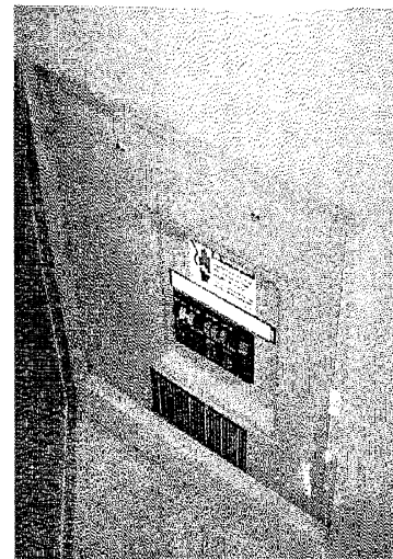
House 110-volt Breaker Panel
