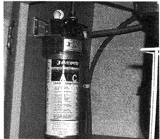
Water Filter Assembly - Below Galley Sink
