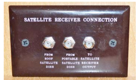
Interior Connection for Satellite Dish (Located in front overhead cabinet) -Typical View
