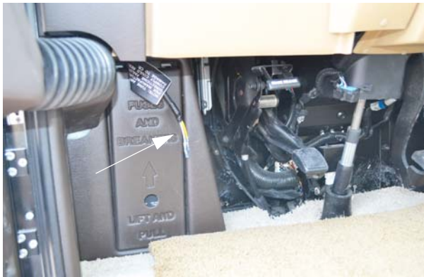
CB Power Wires (Located behind fuse and breaker panel) -Typical View
