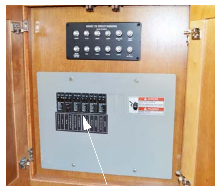
120-Volt House Circuit Breakers -Typical View
