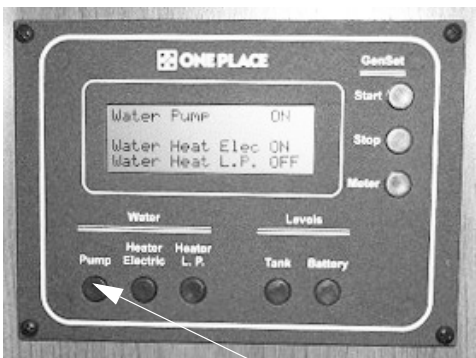
Water Pump Switch
