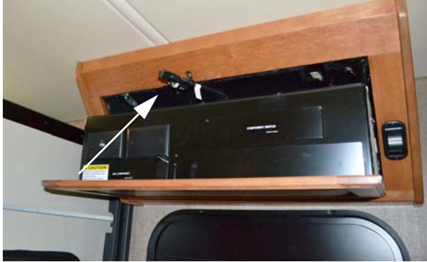
HDMI Cable (Located in cabinet above entrance door) -Typical View
