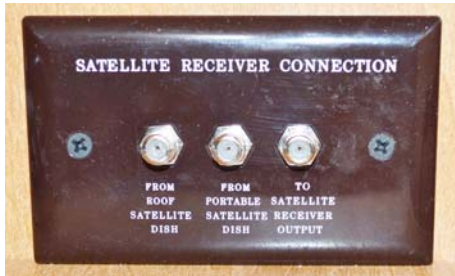
Interior Connection for Satellite Dish (Located in front overhead cabinet) -Typical View
