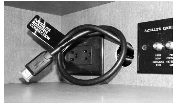
HDMI Cable (Located in cabinet near TV) -Typical View
