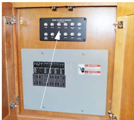
House 12V Breakers -Typical View
