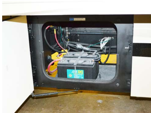
House Batteries (located behind a driver side exterior door) -Model D36Z
