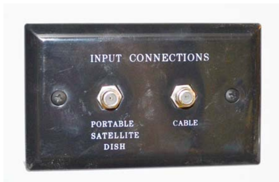
Exterior Connections for Cable TV and Satellite Dish (Located in water service center) -Typical View
