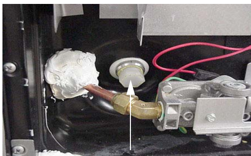
Water Heater Drain Plug (Remove with socket)
