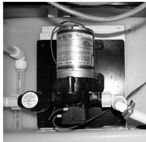
Water Pump (Located inside driver side compartment behind rear wheel) -Typical installation shown
