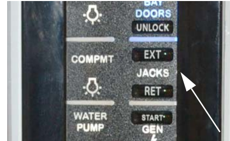
Auto Level Remote Switch (Located near entrance door and/or inside exterior service center)
