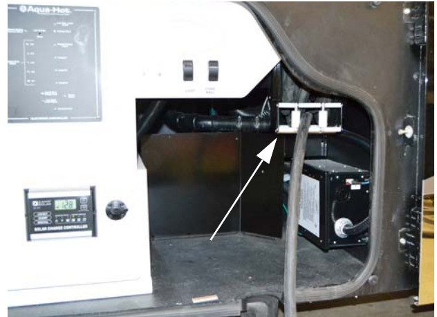
Power Cord Reel (Located in a driver side compartment) -Typical View
