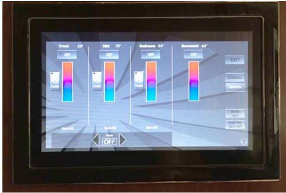
Basement Temperature Control (Located on touch tablet)
