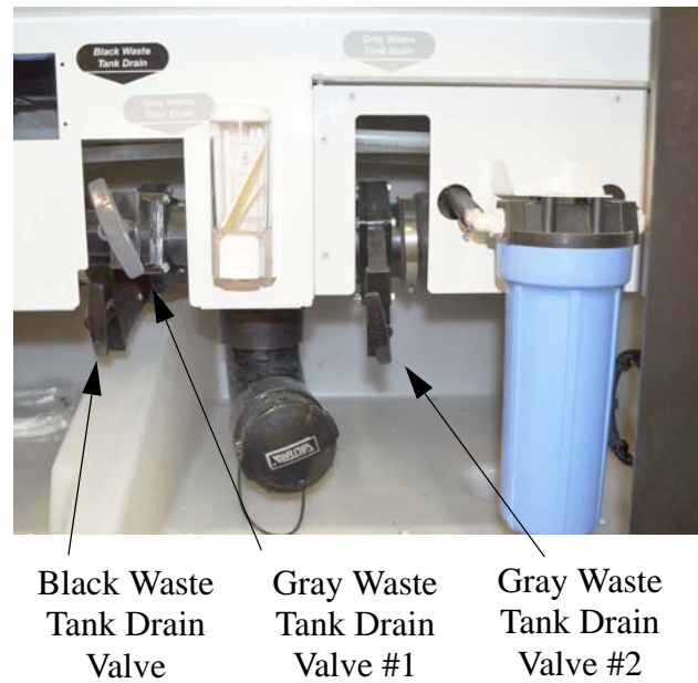
Black and Gray Waste Tank Drain Valves (Located in water service center)
