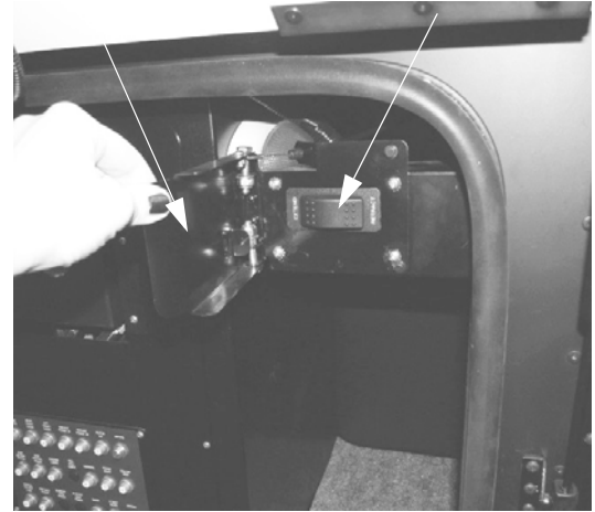
Generator Tray Power Switch and Cover (Located in front driver side compartment)
