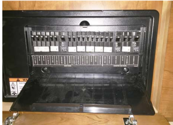
House Circuit Breakers -Typical Installation
