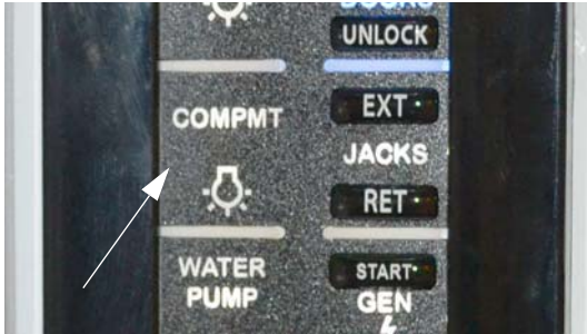
Compartment Lights Switch (Located near entrance door and/or inside a driver side compartment) -Typical View
