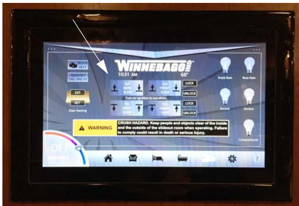
Slideout Room Switches
