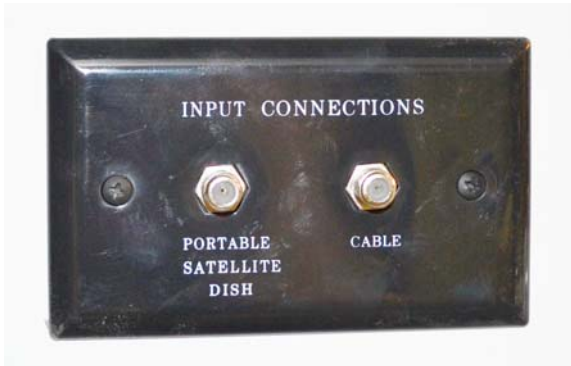
Exterior Connection for Satellite Dish and Cable TV (Located in the shoreline compartment)
