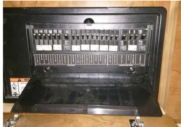
House Circuit Breakers -Typical View
