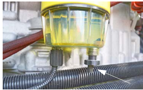
Fuel/Water Separator Drain Valve (Located on bottom end of separator) -Typical View
