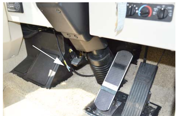
CB Power Wires -Typical View
