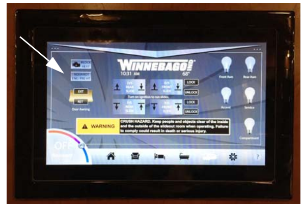
Hydronic Heating System Interior Control Switches (Located on touch tablet “Exterior” screen)
