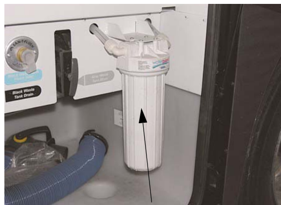
Full-Coach Water Filter System (Located in water service center) -Typical View
