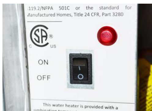
Water Heater (Tankless) Power Switch
