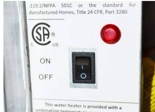
Water Heater (Tankless) Power Switch
