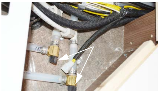
Waterline Drain Valve
