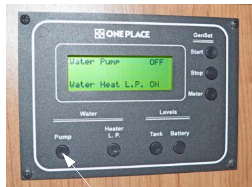
Water Pump Switch
