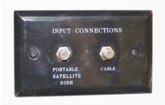
Exterior Connection for Satellite Dish and Cable TV (Located in the shoreline compartment)
