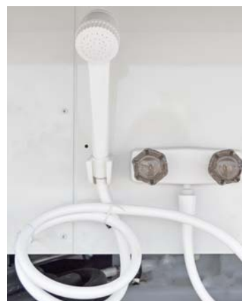
Exterior Shower/Wash Station -Typical View
