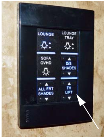
Buffet TV Power Lift/Lower Control Switch (Located near sofa) -Typical View
