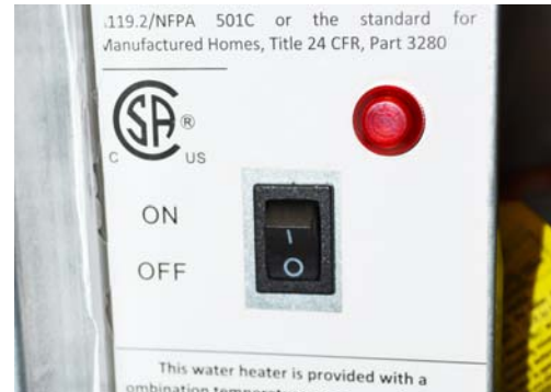
Water Heater (Tankless) Power Switch
