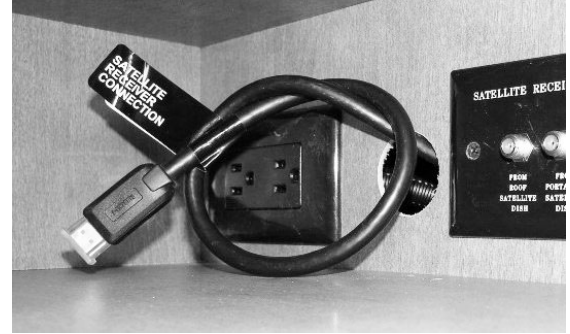
HDMI Cable (Located near entertainment center cabinet) -Typical View
