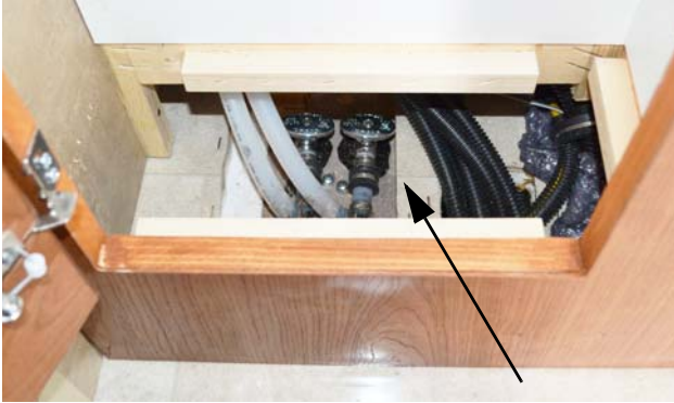
Waterline Drain Valves -Typical installation shown
