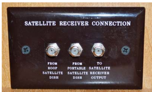
Interior Connection for Satellite Dish (Located near entertainment center cabinet) -Typical View
