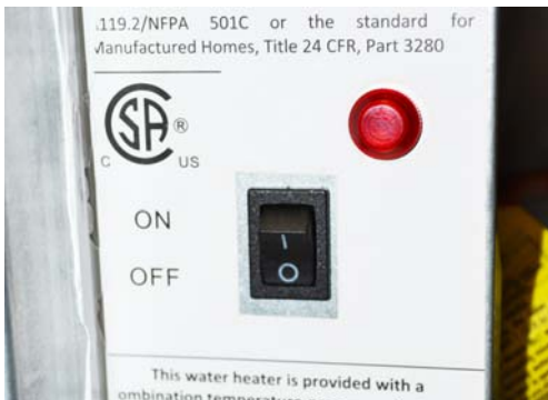
Water Heater (Tankless) Power Switch
