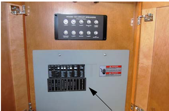
120-Volt House Circuit Breakers -Typical View
