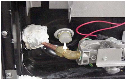
Water Heater Drain Plug (Remove with socket)
