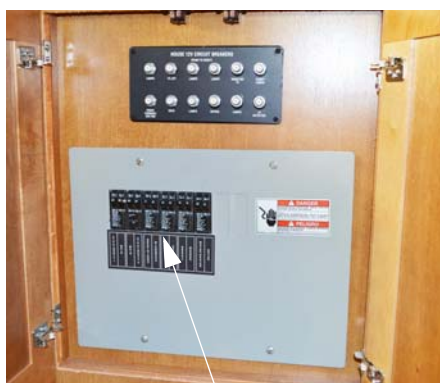
120-Volt House Circuit Breakers -Typical View
