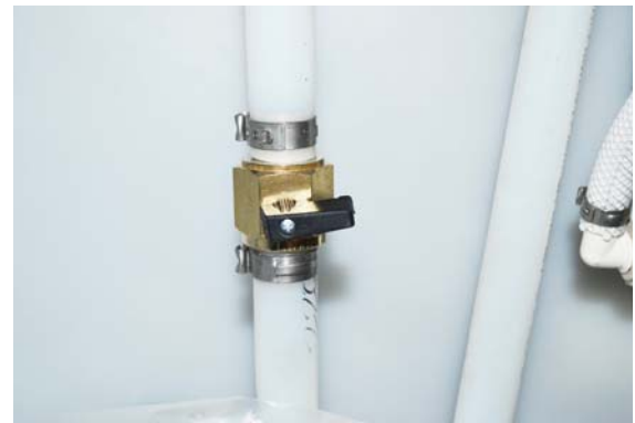
Water Tank Drain Valve -Typical installation shown
