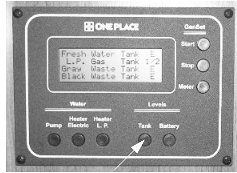
Tank Levels Switch
