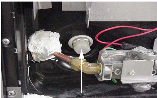
Water Heater Drain Plug (Remove with socket)
