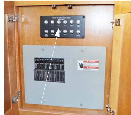
House 12V Breakers -Typical View
