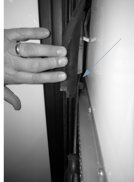
Slideout Motor (Located behind slideout wipe seal)
