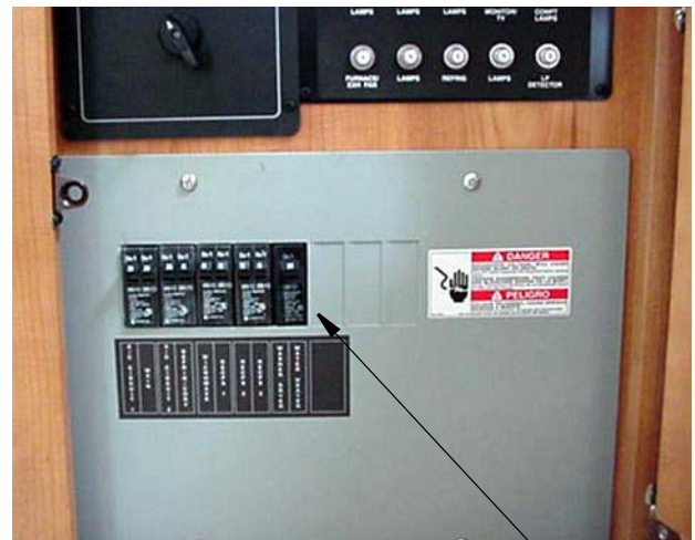
120-Volt House Circuit Breakers -Typical View
