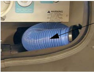
Sewage Drain Hose -Typical View
