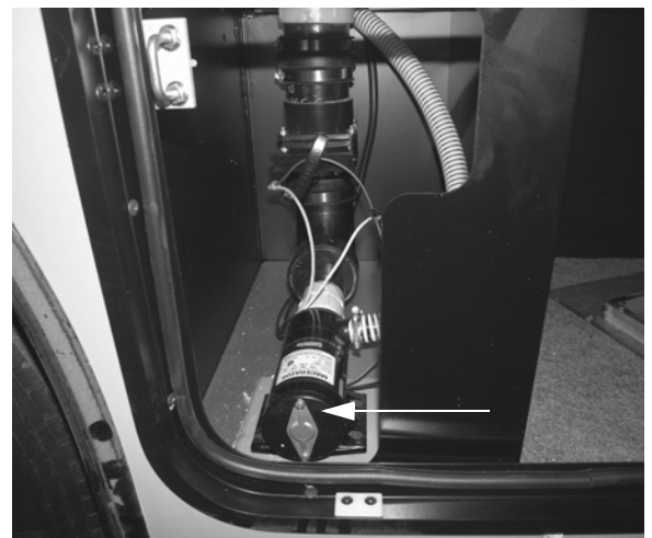
Waste Pump (Located in passenger side compartment ahead of rear axle) -Typical installation shown
