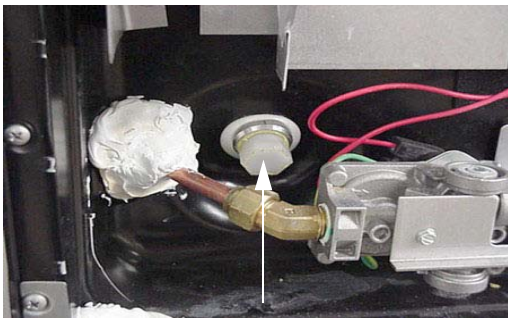
Water Heater Drain Plug (Remove with socket)
