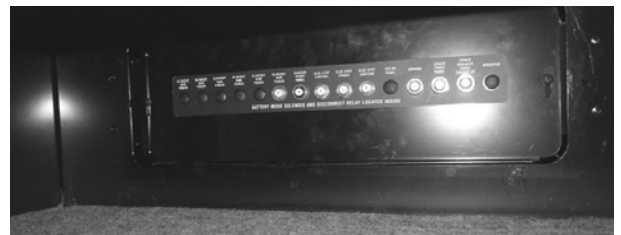
Automotive Chassis and House 12-Volt Circuit Breakers (Located inside passenger compartment) -Typical View
