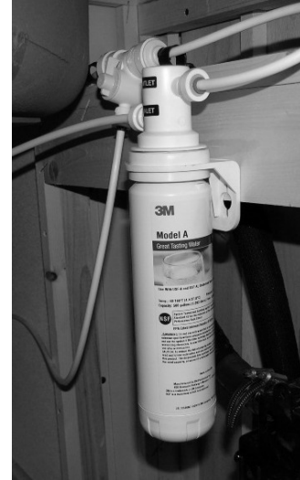
Water Filter Assembly (Located below galley sink) -Typical View
