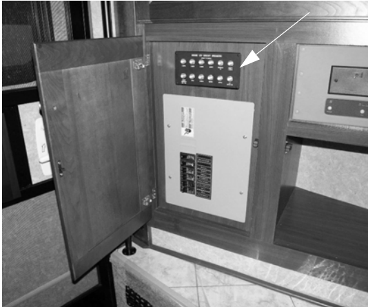
House 12-Volt Circuit Breaker Panel -Typical View
