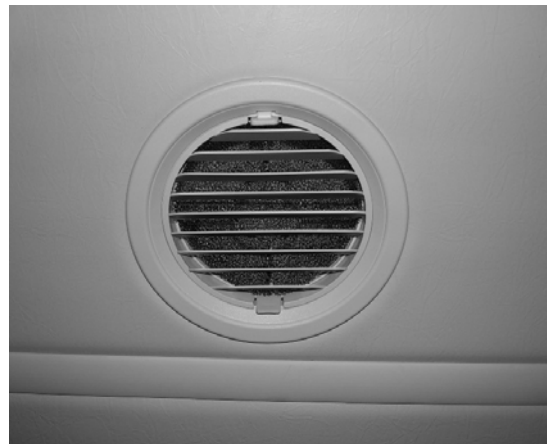
Return Air Vent (Shown with filter installed) -Typical View
