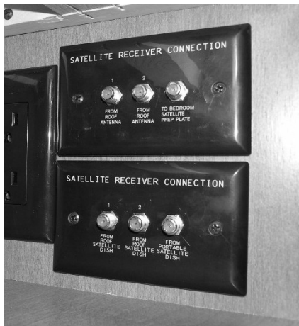
Interior Satellite Dish Connections (Located in the entertainment center cabinet) -Typical View
