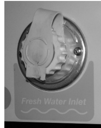
Fresh (City) Water Connection “Fresh Water Inlet” (Located in the water service center)
