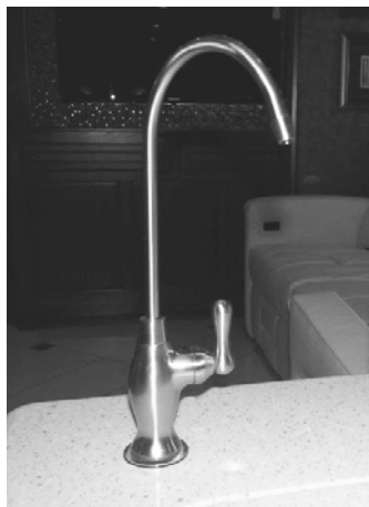
Filtered Water Faucet -Typical View
