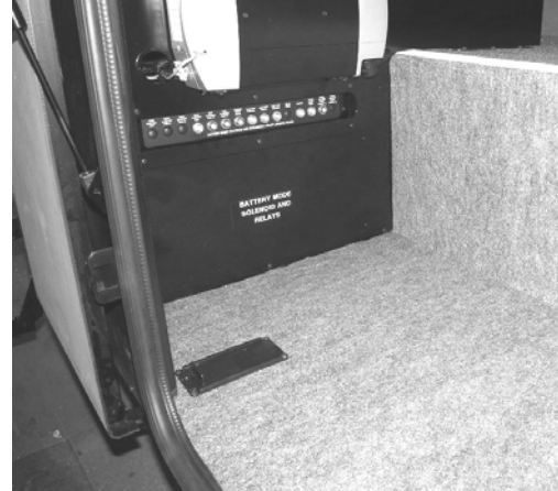
Automotive Chassis and House 12-Volt Circuit Breaker Panel (Located inside passenger compartment) -Typical View
