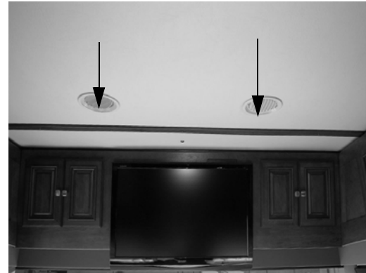
Supply/Return Air Vents (Located throughout the ceiling of the coach) -Typical View
