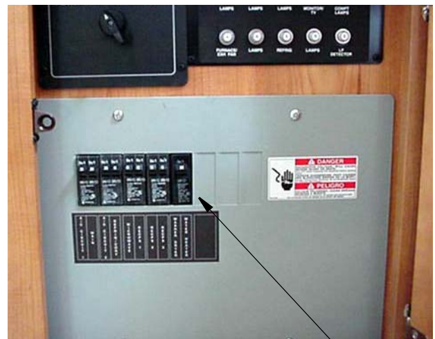
120-Volt House Circuit Breakers -Typical View
