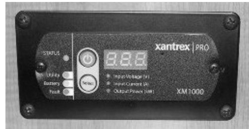
Inverter Control Panel (Located near monitor panel) -Typical View
