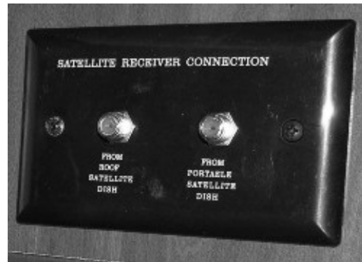
Interior Connection for Satellite Dish (Located in cabinet near TV) -Typical View
