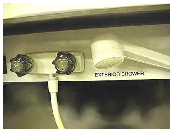
Exterior Shower/Wash Station -Typical View
